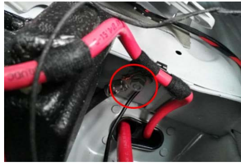
14. Position of negative pole iron of power supply
