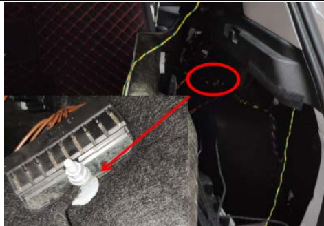
15. Position of negative pole iron of power supply
